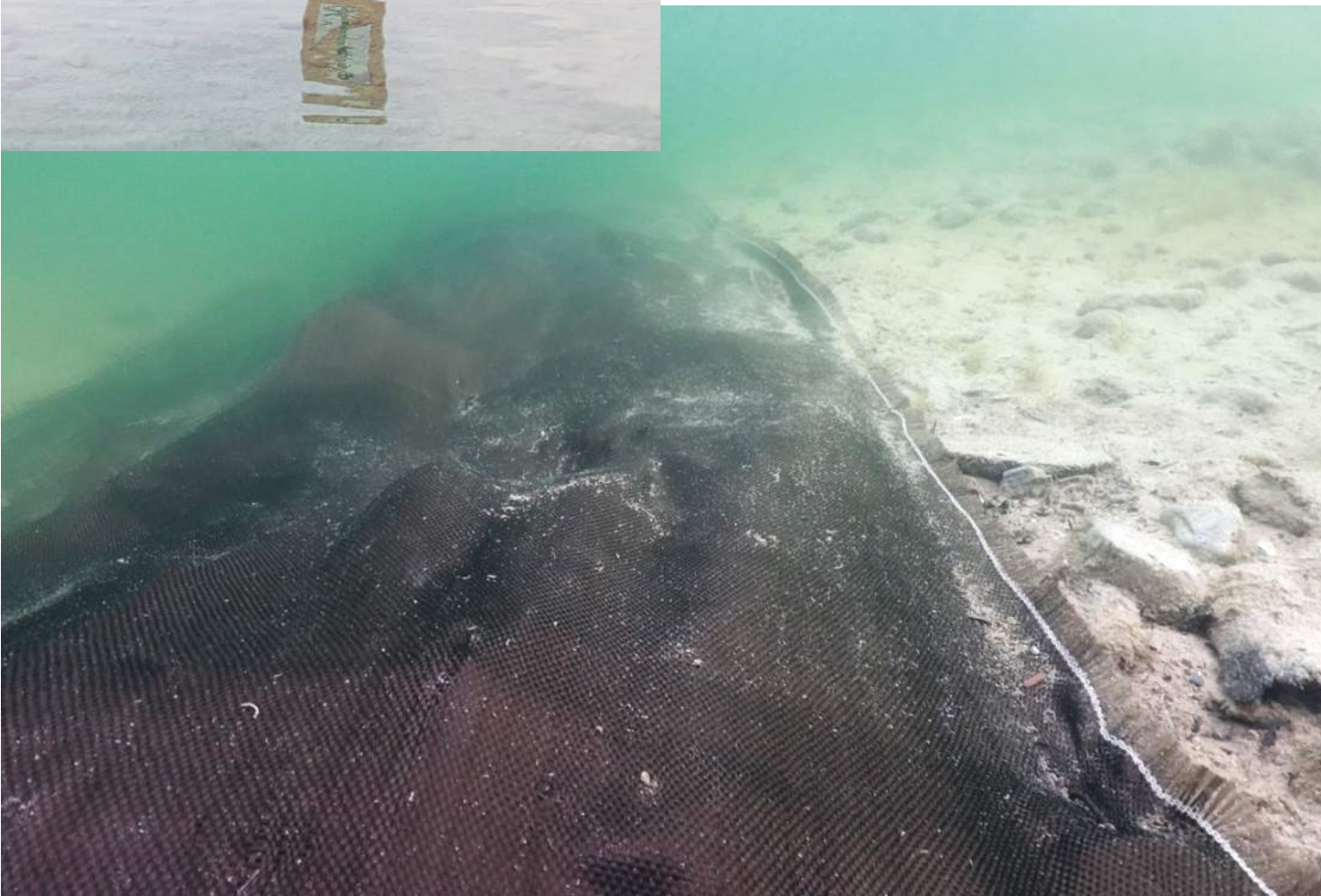
Erosionsschutzmatte aus Basalt, Mondsee Erosion protection mat made of basalt, Lake Mondsee
